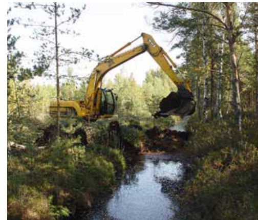
Fig. 17.6. Construction of peat dam with excavator on the side of Great Ķemeri Mire. Photo: J. Kuze.
