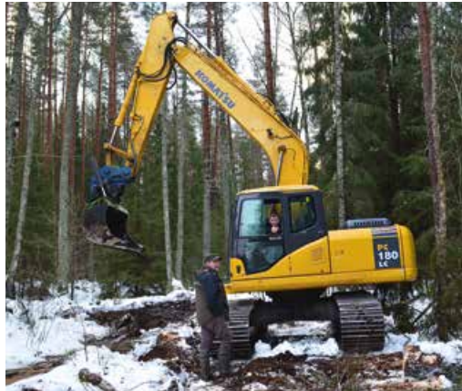
Fig. 17.10. Filling of a ditch with an excavator in Gauja National Park. Photo: S. Ikauniece.
