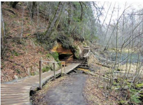
Fig. 11.21. A boardwalk (before renovation) along Sarkanās klintis ( Red Cliffs ) near Cēsis had become unsafe (it was slippery, plank ends were moving, there were no boundary railings), therefore visitors took the opportunity to walk next to the boardwalk and trampled the basal part of the outcrop. Photo: I. Čakare.
