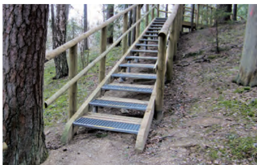
Fig. 11.30. Stairs with metal steps, which will serve for a long time, are constructed in Estonia at Tevaskoje outcrops. Photo: I. Čakare.
