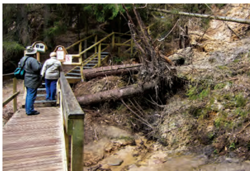
Fig. 11.28. Stair strengthening was planned on a sandstone outcrop in Estonia at the River Ahja, but the construction of a stair buttress in a spring discharge site caused a landslide. It indicates that careful investigation of the ground before the construction of infrastructure is an important part in the planning of trails. Photo: I. Čakare.
