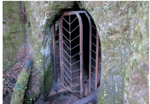
Fig. 12.8. Incorrectly constructed bars in Līgatne. Crossbars are inclined, rather than straight. Photo: I. Čakare.
