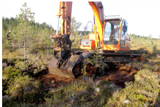
Fig. 10.20. It is recommended to use peat for the filling up of ditches, taken from the bog surface by excavator, forming shallow depressions. It can be expected that they will overgrow with bog vegetation within a few years. Photo from the bog restoration site in Finland. Photo: I. Lazda.
