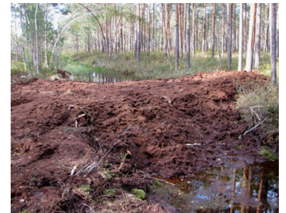
Fig. 2.10. A recently built peat dam on the ditch in Rožu Bog in 2013. Photo: A. Priede.
