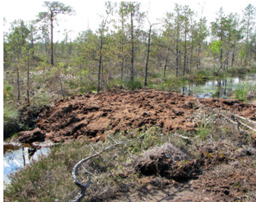
Fig. 10.39. Recently installed peat dam, built with an excavator in Rožu Bog. The dam surface is higher than the bog surface, taking into account the compaction of peat. Photo: A. Priede.
