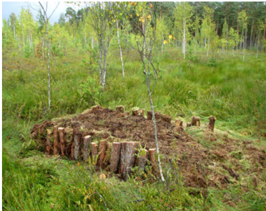
Fig. 10.38. Manually built peat dam in 2013 in Aizkraukle Bog on a small, almost overgrown ditch. The edges of the dam are reinforced with wooden piles. Photo: A. Priede.
