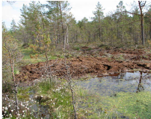
Fig. 10.41. A peat dam built with an excavator in Rožu Bog (in 2013). Photo: A. Priede.
