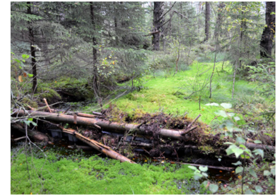
Fig. 10.35. A plastic piling dam masked with fallen logs and branches in Kamanos Strict Nature Reserve in Lithuania. Photo: S. Ikauniece.
