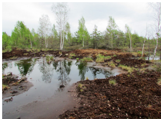
Fig. 10.42. For the construction of the dam in Lake Melnais Bog, the peat was obtained from the bog surface near the dam, creating a shallow pond. The photo was taken a year after the installation of the dam. It is expected that in the longer term the depression will overgrow with quaking bog vegetation. Photo: A. Priede.
