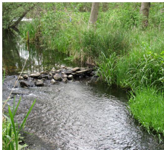
Fig. 15.17. A small boulder threshold in the stream, built to raise the water table in a fen in Brandenburg, Germany. Photo: A. Priede.
