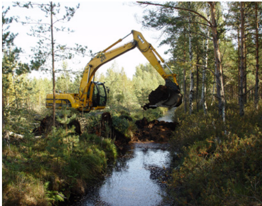
Fig. 10.40. Construction of a peat dam with an excavator in Great Ķemeri Mire in 2006. First, trees along the ditch, which can interfere with excavator movement were felled. Then, a peat dam several metres wide was built by obtaining peat from the adjacent area, thus creating small ponds. Photo: J. Ķuze.
