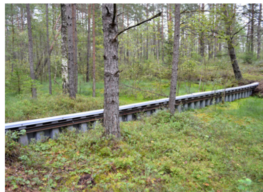
Fig. 10.33. A plastic piling dam built over a wide ditch in Kamanos Strict Nature Reserve in Lithuania. Photo: S. Ikauniece.
