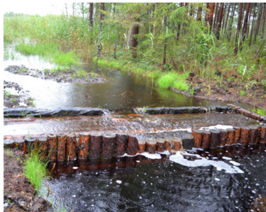
Fig. 10.27. Wooden dam in Soomaa Bog in Estonia consists of two rows of logs driven perpendicular to the ditch, filled with peat. Surface is strengthened with boards, but the upstream of the dam is isolated with durable plastic film. Photo: S. Ikauniece.
