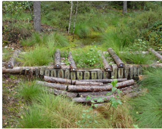
Fig. 10.25. Dam in Teiči Bog, constructed of timber (logs) obtained on site (built in 2003). A few years after the installation, the dam is already overgrown with bog plants. Photo: J. Kuze.
