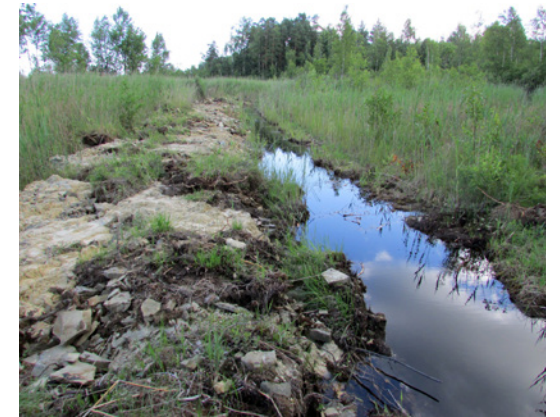
Fig. 14.7. Recently excavated ditch in an alkaline fen with Cladium mariscus on the shore of Lake Kaņieris in 2014. Here, the only habitat-favourable activity is the elimination of this impact by filling up the ditch immediately. In this case, the berm can be used for filling up the ditch. Most probably, alkaline fen vegetation will recover within a few years after filling up the ditches. Photo: A. Priede.
