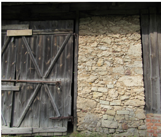
Fig. 2.5. A barn wall built of tufa and limestone pieces in an old farming house near Matkule Village in western Latvia. The rocks are taken from Imula River valley where tufa forms from carbonate-rich springs. Extracting tufa for different usages has depleted most of Ķauķu Hill (Ķauķu kalns, also called Kursas Staburags) that once had a large deposit of tufa. Photo: A. Priede.
