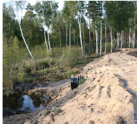
Fig. 10.61. In Great Ķemeri Mire in the former peat extraction site, the road has been used as a dam in order to increase the water level, by raising its surface. The water level is regulated by a culvert. In the photo – the dam during construction works in 2006; the culvert has just been installed, so the water level has not yet risen. Photo: A. Liepa.
