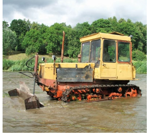
Fig. 17.29. In the River Mūsa, in order to reduce the aquatic plant overgrowth and to scarify the root system, a caterpillar tractor is used. Photo: A. V. Urtāns.
