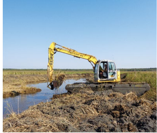
Fig. 13.11. Deepening of a channel to renew water circulation and organism migration. L. Engure.
