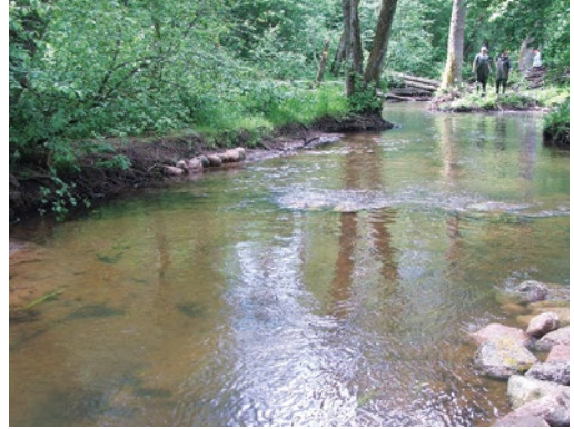
River stretch with installed riffle and bank stabilisation with stone riprap. R. Kauliņa. Photo: L. Urtāne.
