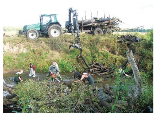
Use of lifting mechanisms to withdraw timber from the river. R. Palsa. Photo: L. Urtāne.
