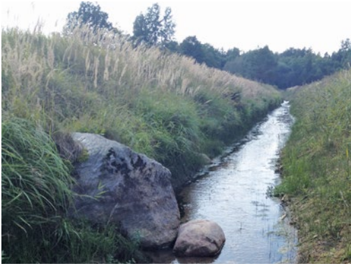
Fig. 17.17. A regulated reach of a fast flowing river with a uniform riverbed. The microhabitat diversity on the riverbed is low. The stone left on the riverbed is used by organisms as a hideout. Photo: A. V. Urtāns.
