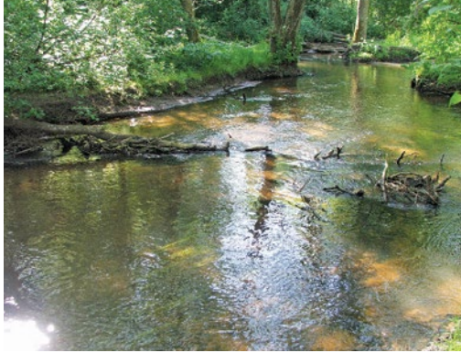
Eroded and widened river before riffle area renewal. R. Kauliņa. Photo: L. Urtāne.
