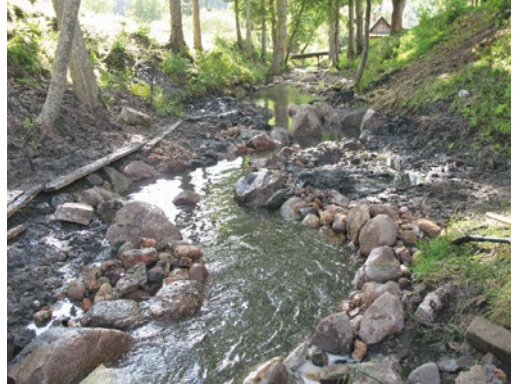
Stone riprap on both banks ensures bank stability, increased stream velocity, scouring of sediments, reopening of the natural gravel channel bed. Photo: A. V. Urtāns.
