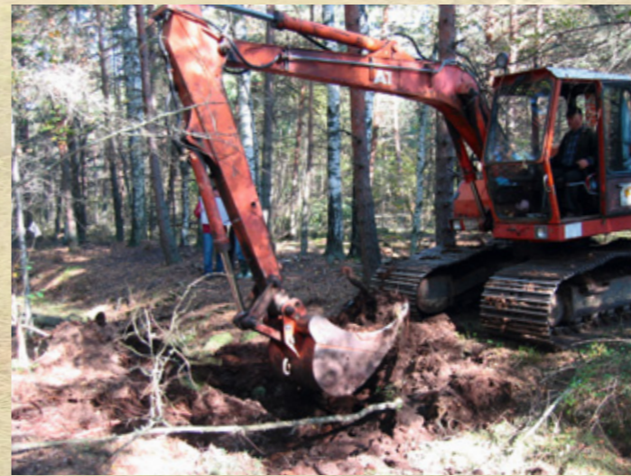
Photo: V. Baroniņa Building of peat dams on drainage ditches on the raised bog margin.
